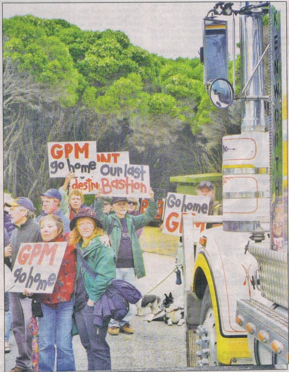
Work started on a new ocean access boat ramp at Mallacoota on Monday, with construction workers greeted by protestors from the Save Bastion Point group. One protestor is reported to have sat down in front of a truck that arrived on scene, with others gathering around in support. (PS)
