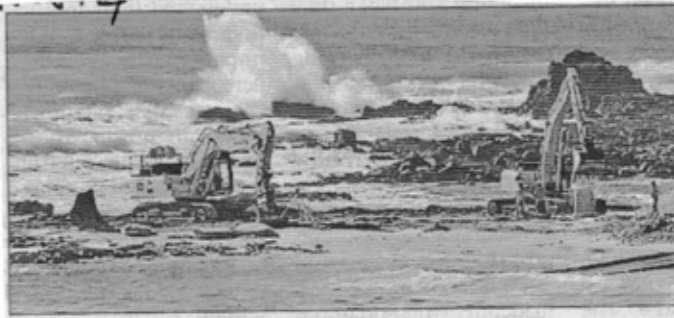
• Construction of a new two lane boat ramp at Mallacoota began on Monday. Photograph by Michael Rayner.
